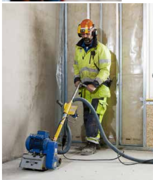
Suction is available on each floor.
